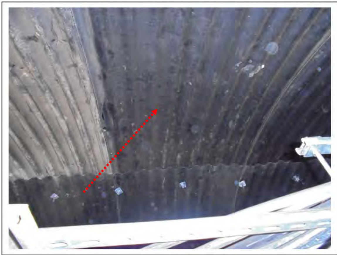
FIGURE 79: CONFIRMED ASBESTOS IN CELLACTITE SHEETING IN SWITCH ROOM, 5/661 - DESCRIPTION & RESULT OF ASSESSMENT (SAMPLE REF. ECS 85278)
