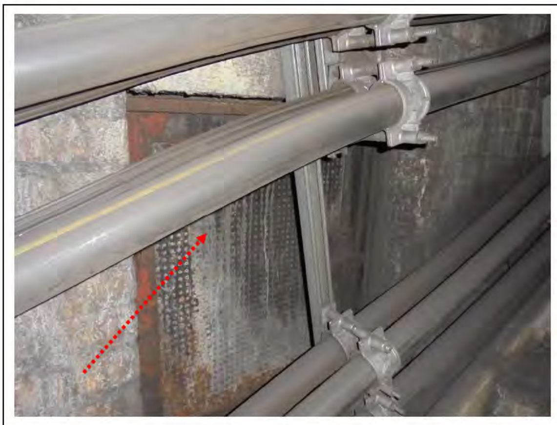
FIGURE 37: CONFIRMED ASBESTOS IN DURASTEEL PANEL IN CABLE TUNNEL, 4/786 - DESCRIPTION & RESULT OF ASSESSMENT (SAMPLE REF. AS 014003/18)
