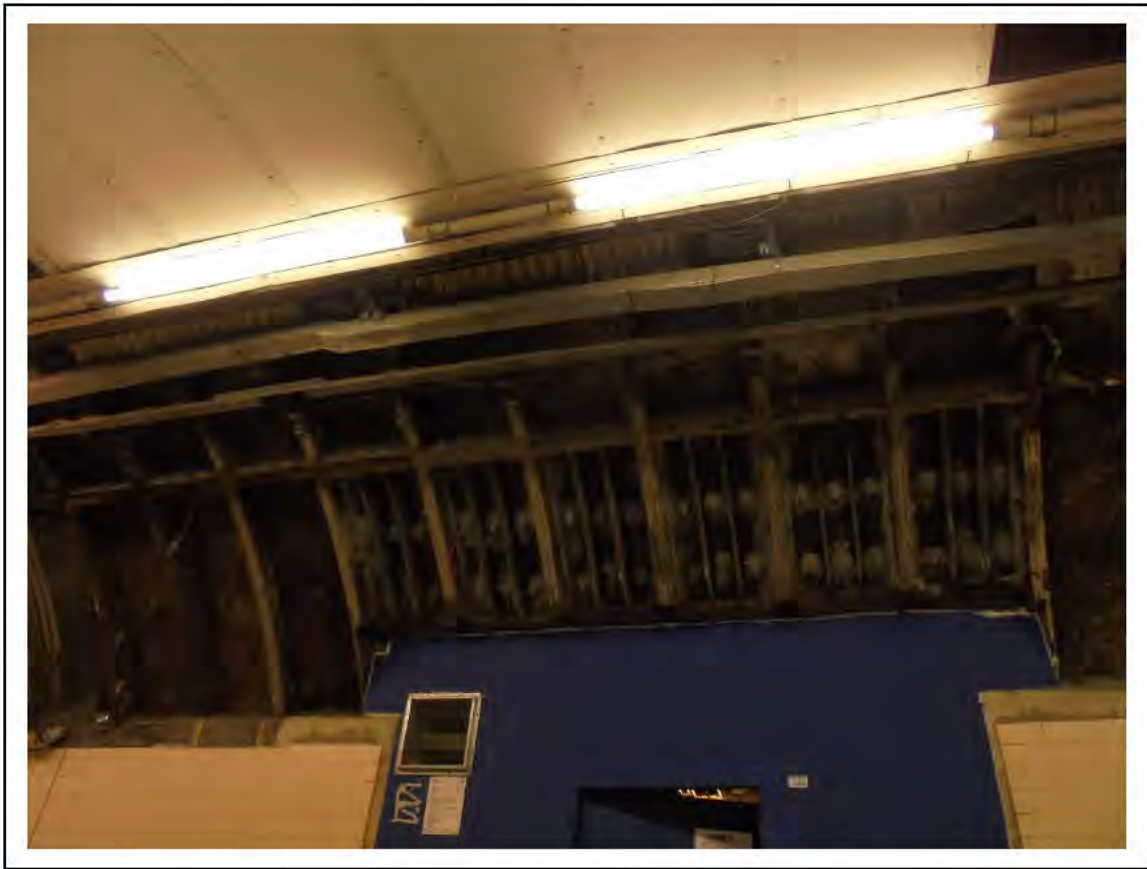
FIGURE 67: CONFIRMED ASBESTOS IN TUNNEL RING CAULKING IN CIRC AREA, 4/091 - DESCRIPTION & RESULT OF ASSESSMENT (SAMPLE REF. AS 014003/12)
