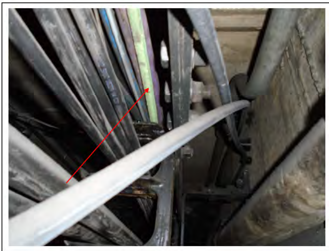
FIGURE 29: KNOWN ASBESTOS IN WOVEN CABLE INSULATION IN LMC 3, 4, 5 CRAWLWAY, 6/161 - DESCRIPTION & RESULT OF ASSESSMENT (SAMPLE REF. K1 (4))
