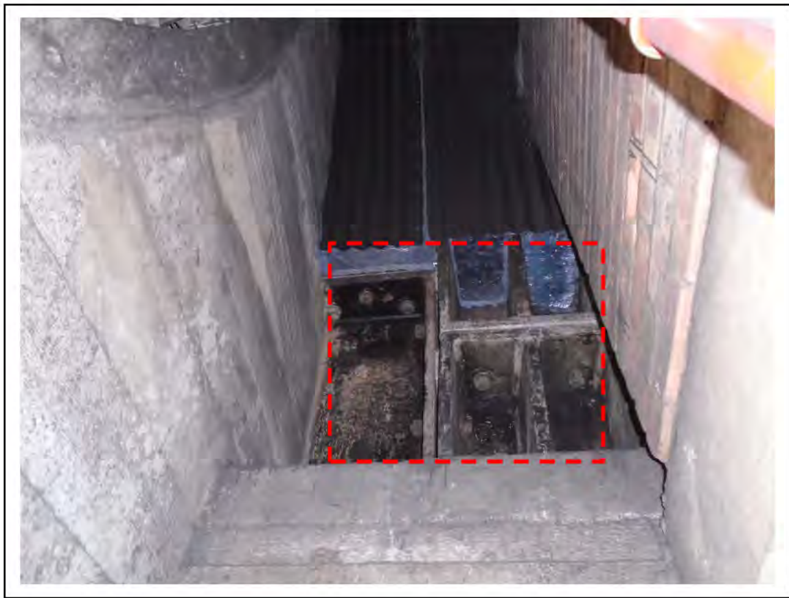
FIGURE 24: CONFIRMED ASBESTOS IN TUNNEL RING CAULKING IN LMC 3, 4, 5, 6/161 - DESCRIPTION & RESULT OF ASSESSMENT (SAMPLE REF. 100558/141010/1)
