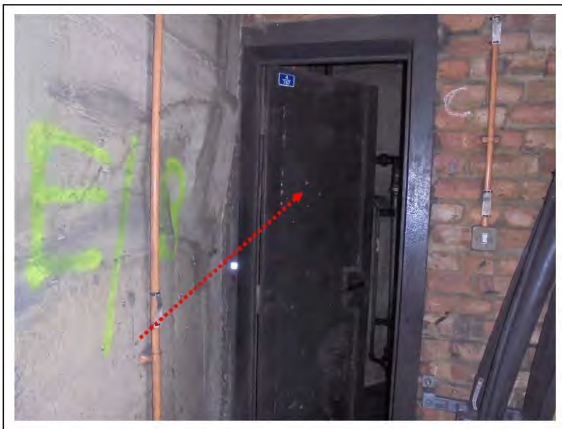
FIGURE 34: CONFIRMED ASBESTOS IN DURASTEEL PANEL IN CABLE TUNNEL, 4/786 - DESCRIPTION & RESULT OF ASSESSMENT (SAMPLE REF. ECS 76821)
