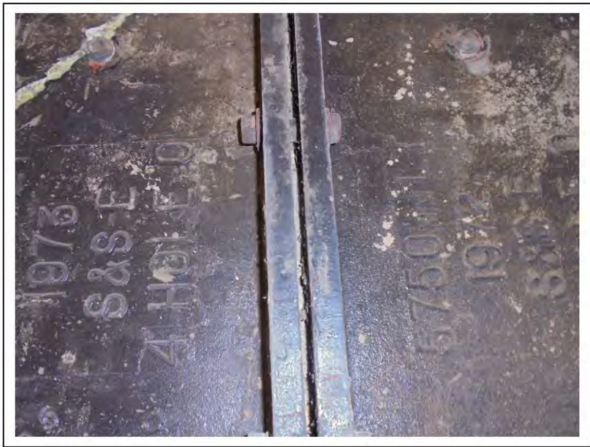
FIGURE 69: CONFIRMED ASBESTOS IN TUNNEL RING CAULKING IN PASSAGE, 4/204 - DESCRIPTION & RESULT OF ASSESSMENT (SAMPLE REF. 100675/231110/5)
