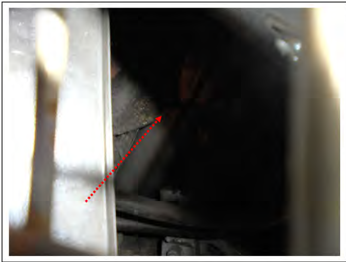
FIGURE 68: CONFIRMED ASBESTOS IN CELLACTITE SHEETING IN CIRC AREA, 4/091 - DESCRIPTION & RESULT OF ASSESSMENT (SAMPLE REF. 110452/160811/01)
