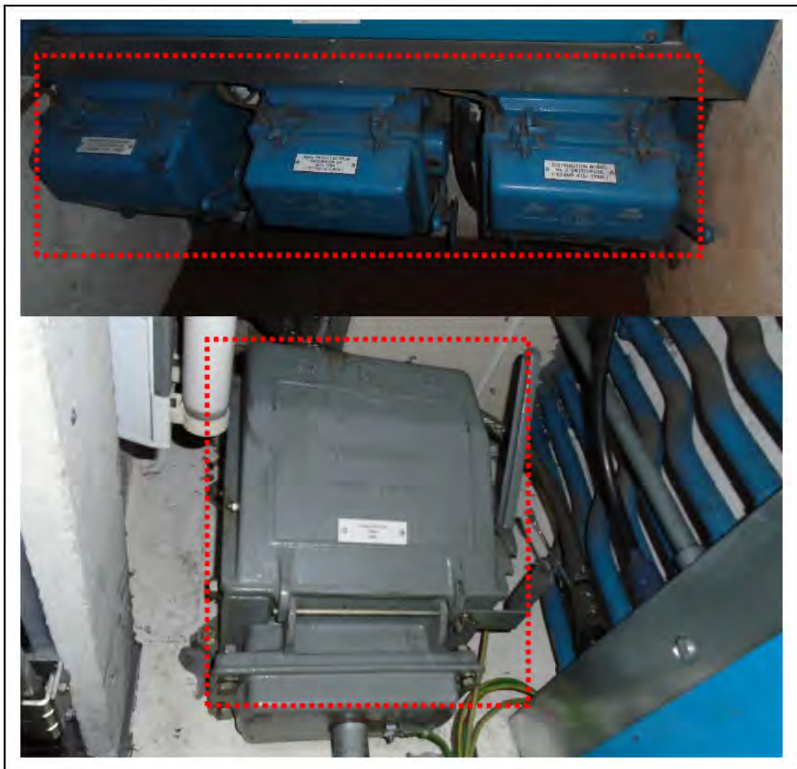
FIGURE 10: STRONGLY PRESUMED ASBESTOS IN COMBINATION FUSE SWITCHES IN SWITCHROOM E3, 2/663 - DESCRIPTION & RESULT OF ASSESSMENT (SAMPLE REF. SP1 (3))
