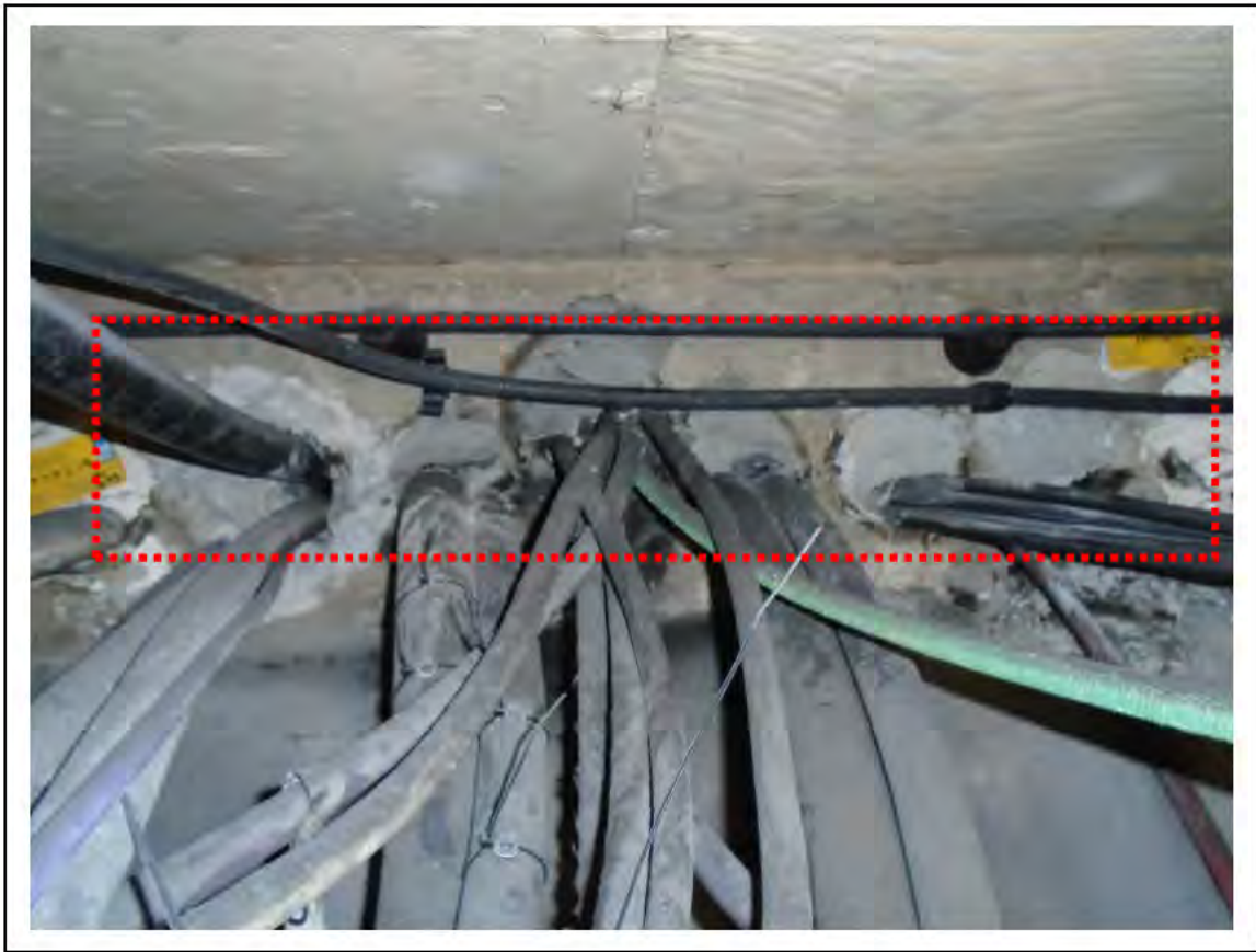
FIGURE 31: CONFIRMED ASBESTOS IN BITUMEN DUCTS IN LMC 3, 4, 5 CRAWLWAY, 6/161 - DESCRIPTION & RESULT OF ASSESSMENT (SAMPLE REF. 161144/190916/11)
