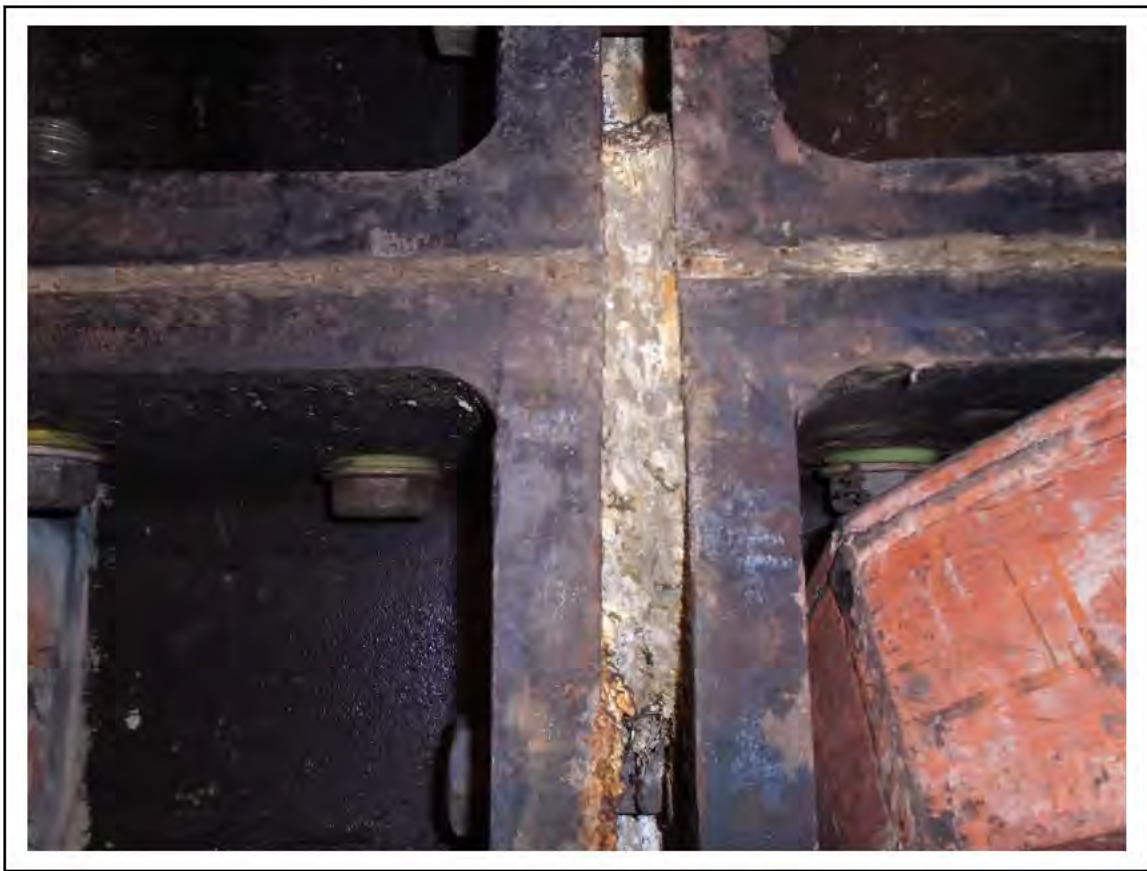
FIGURE 33: CONFIRMED ASBESTOS IN TUNNEL RING CAULKING IN STORE, 4/571 - DESCRIPTION & RESULT OF ASSESSMENT (SAMPLE REF. 100558/131010/5)
