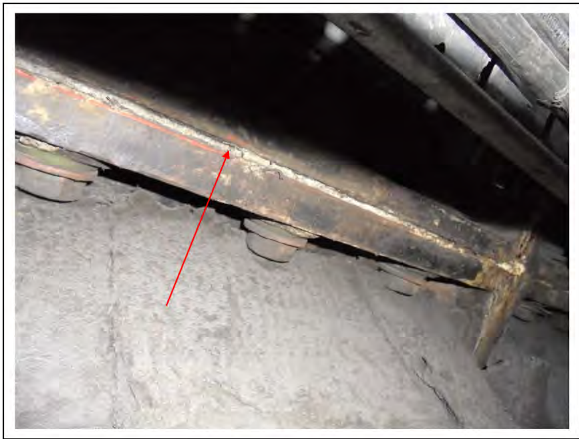
FIGURE 64: CONFIRMED ASBESTOS IN TUNNEL RING CAULKING IN PASSAGE, 4/205 - DESCRIPTION & RESULT OF ASSESSMENT (SAMPLE REF. ECS85389)
