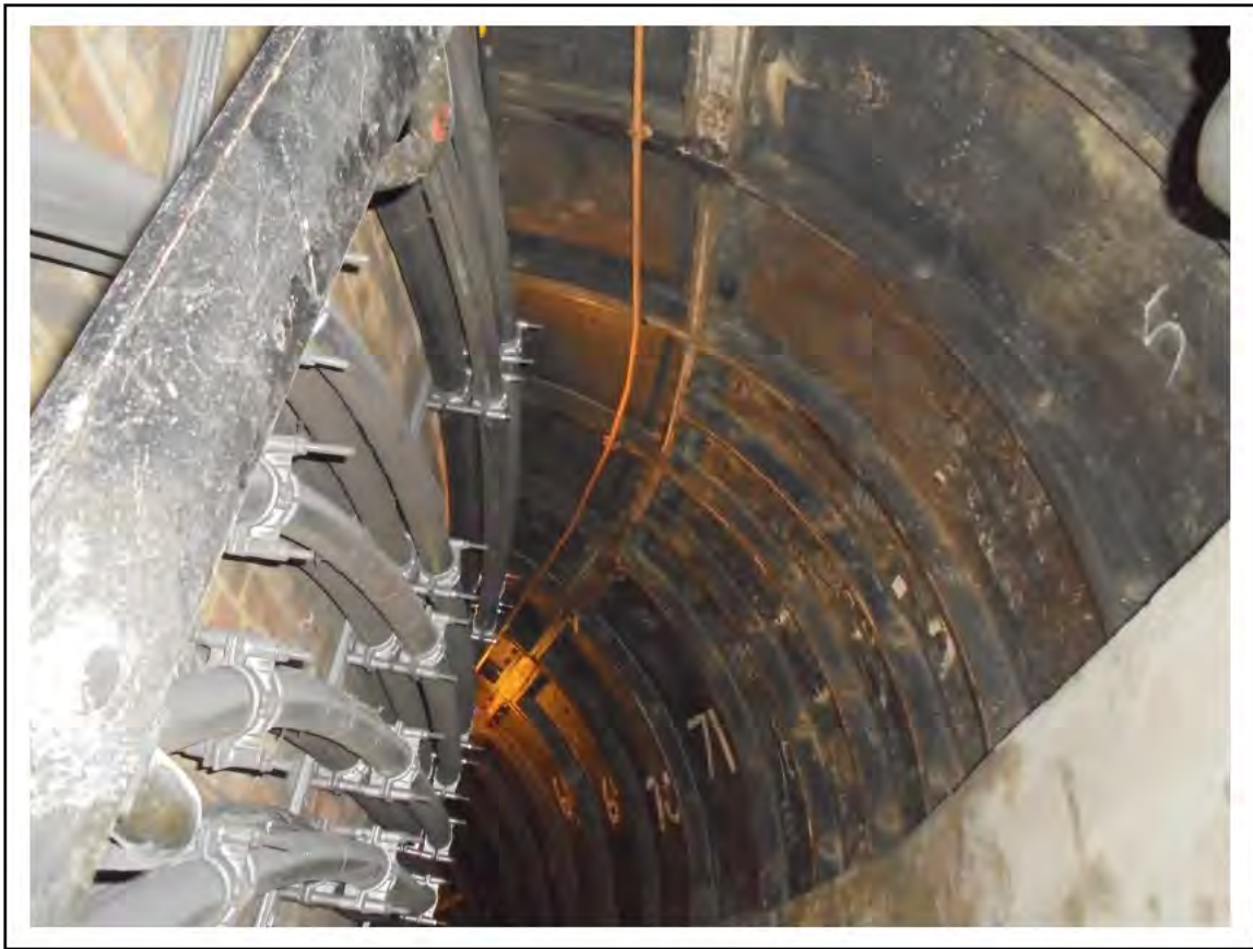
FIGURE 36: CONFIRMED ASBESTOS IN CAULKING IN CABLE TUNNEL, 4/786 - DESCRIPTION & RESULT OF ASSESSMENT (SAMPLE REF. ECS 85380)
