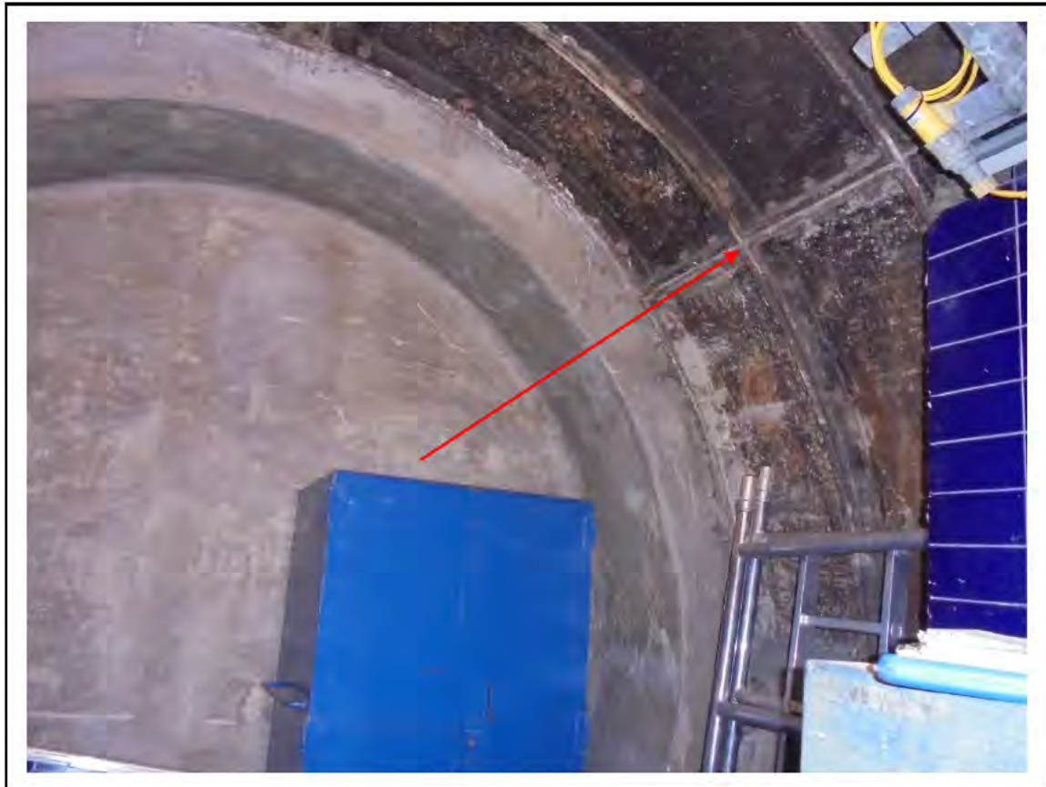
FIGURE 55: CONFIRMED ASBESTOS IN CAULKING TO CAST IRON TUNNEL RINGS IN PASSAGE (BLOCKED OFF BOTH ENDS), 6/208 - DESCRIPTION & RESULT OF ASSESSMENT (SAMPLE REF. 110714/071111/05 & 06)
