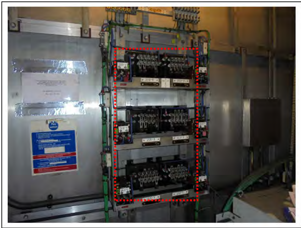
FIGURE 91: STRONGLY PRESUMED ASBESTOS IN OLD SILUMINITE BACKING PANELS IN RELAY ROOM, 6/711 - DESCRIPTION & RESULT OF ASSESSMENT (SAMPLE REF. SP1 (12))
