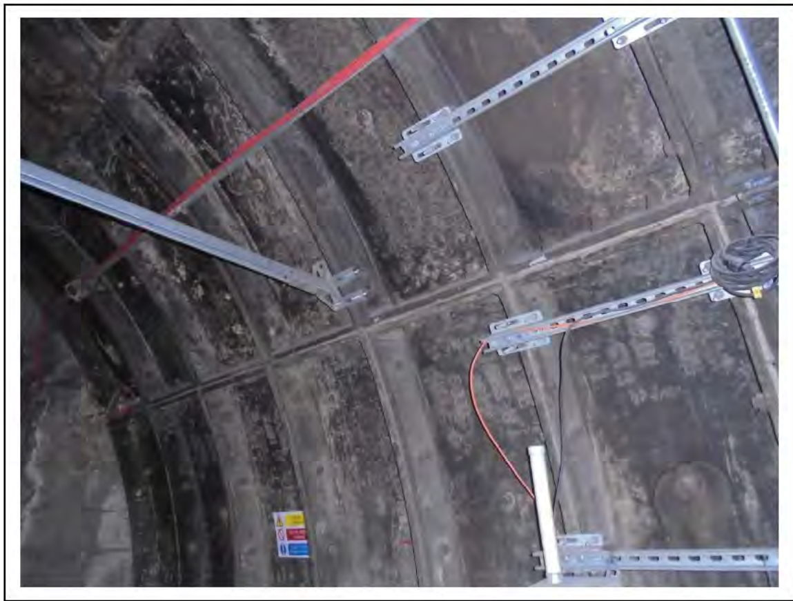
FIGURE 52: CONFIRMED ASBESTOS IN CAULKING TO TUNNEL RINGS IN DRAFT RELIEF TUNNEL, 6/792 - DESCRIPTION & RESULT OF ASSESSMENT (SAMPLE REF. ECS 85356)
