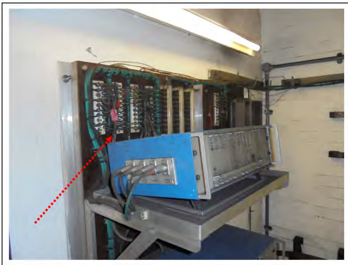
FIGURE 81: PRESUMED ASBESTOS IN BROWN COMPOSITE SILUMINITE BOARDS IN RELAY ROOM, 5/712 - DESCRIPTION & RESULT OF ASSESSMENT (SAMPLE REF. P1 (2))
