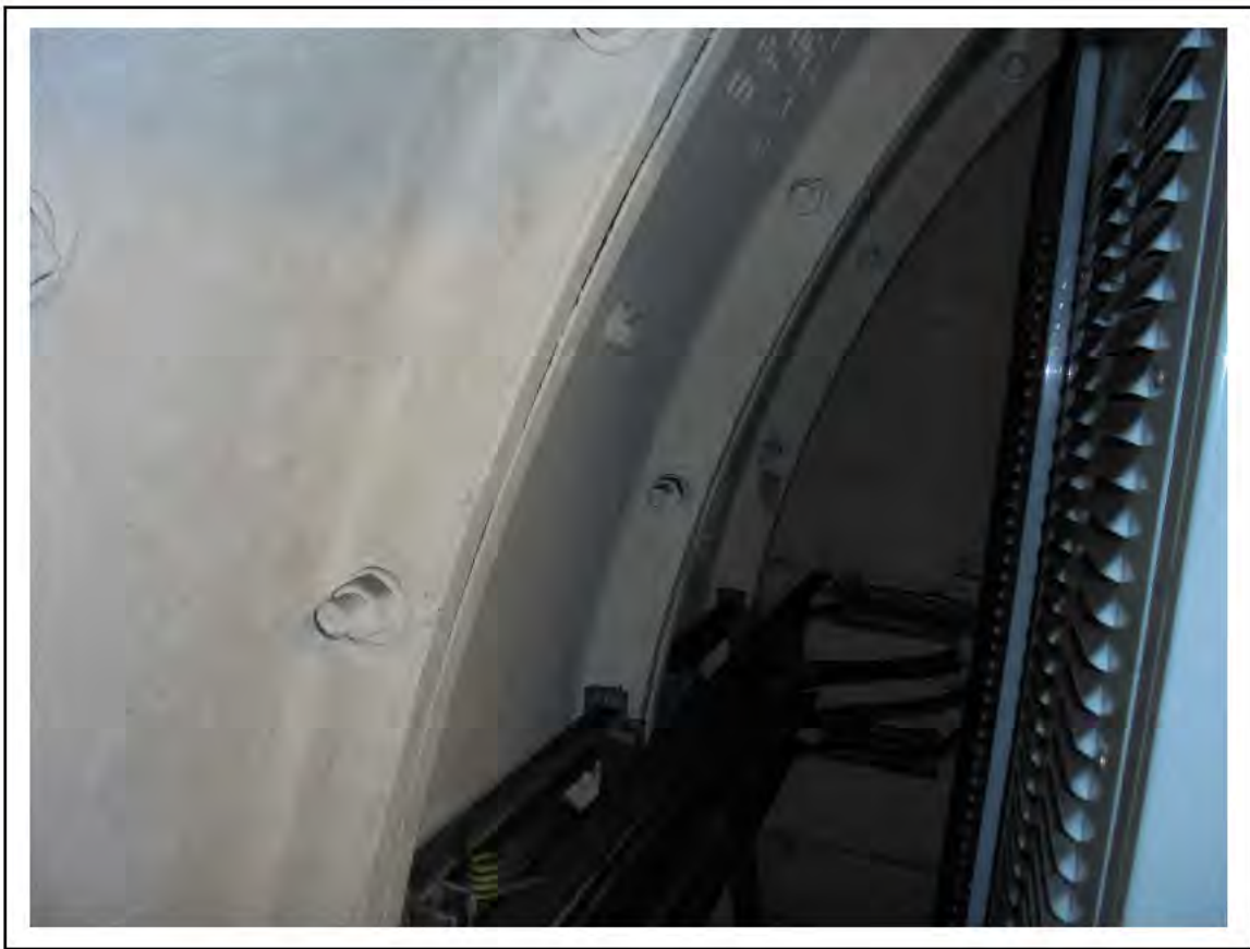
FIGURE 90: CONFIRMED ASBESTOS IN CAULKING IN SWITCH CUPBOARD E9, 6/662 - DESCRIPTION & RESULT OF ASSESSMENT (SAMPLE REF. ECS 85356)
