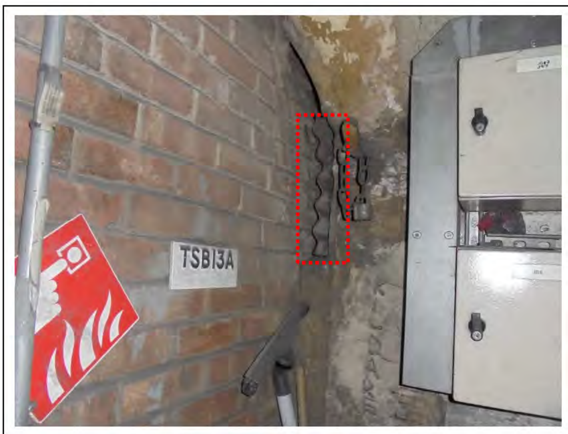
FIGURE 43: CONFIRMED ASBESTOS IN CELLACTITE IN VENT TUNNEL, 4/794 - DESCRIPTION & RESULT OF ASSESSMENT (SAMPLE REF. ECS 76827)
