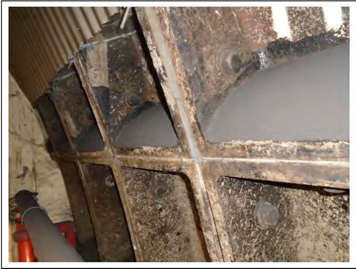
FIGURE 12: CONFIRMED ASBESTOS IN TUNNEL RING CAULKING IN UMC 3,4,5 LOBBY TO CHAMBER, 4/161 - DESCRIPTION & RESULT OF ASSESSMENT (SAMPLE REF. 100558/121010/8)
