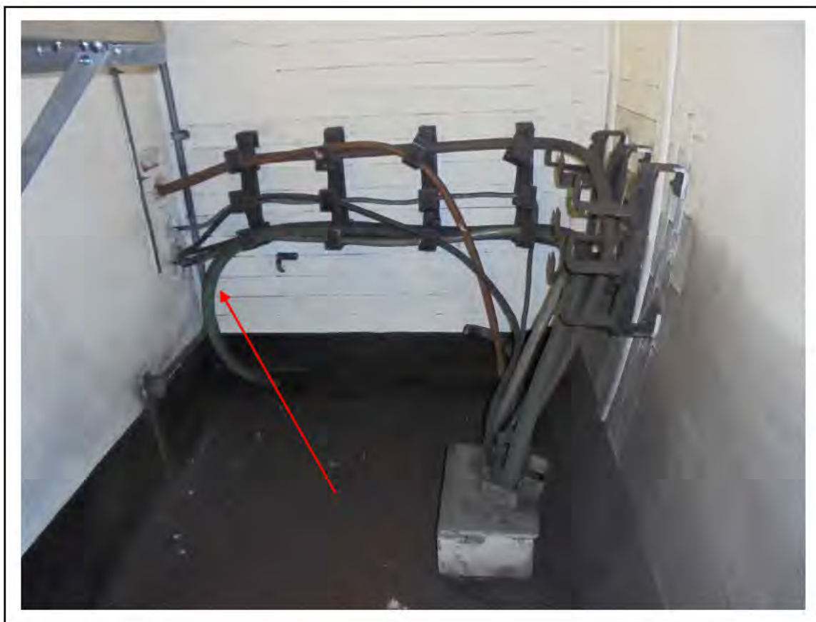
FIGURE 80: CONFIRMED ASBESTOS IN WOVEN CABLE IN RELAY ROOM, 5/712 - DESCRIPTION & RESULT OF ASSESSMENT (SAMPLE REF. ECS 85274)
