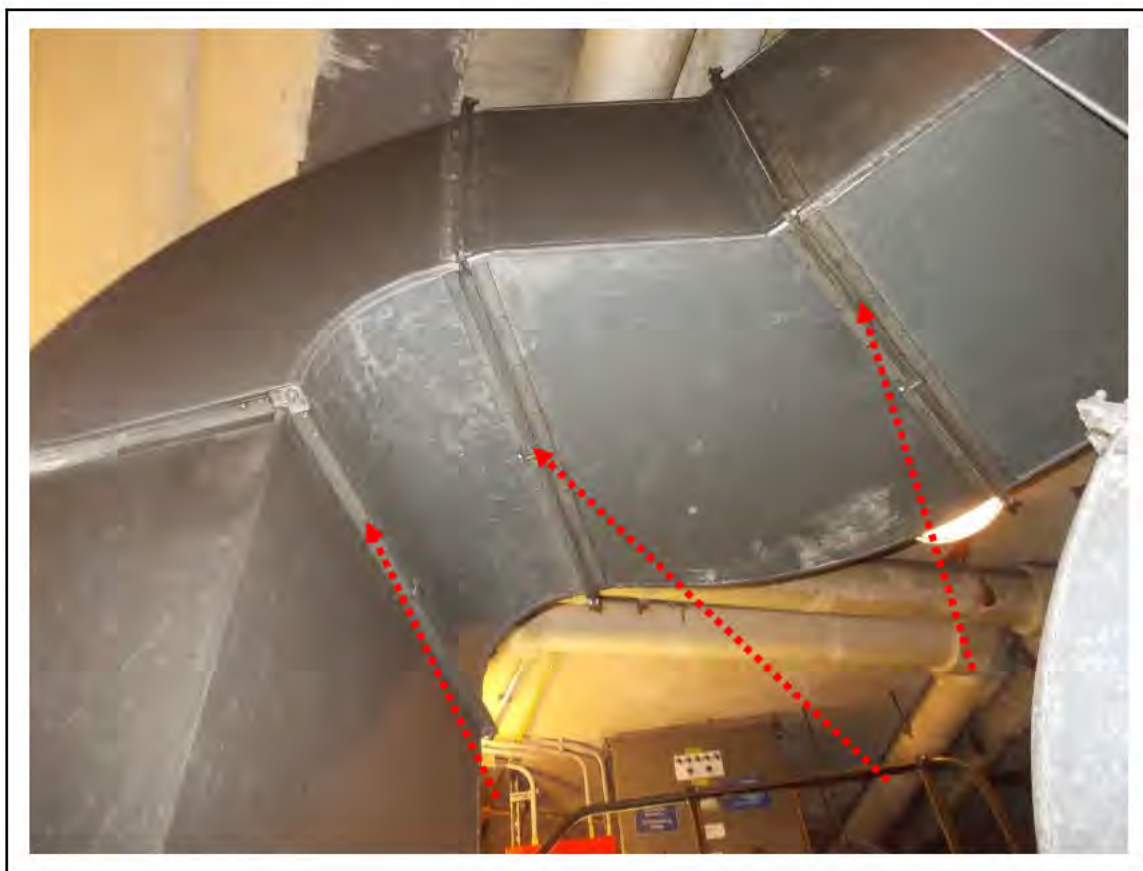
FIGURE 5: CONFIRMED ASBESTOS IN ROPE SEAL IN WORKSITE (FAN ROOM), 2/776 - DESCRIPTION & RESULT OF ASSESSMENT (SAMPLE REF. 014003/10)
