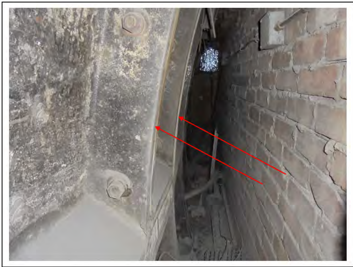
FIGURE 72: CONFIRMED ASBESTOS IN CAULKING TO CAST IRON TUNNEL RINGS IN VENT SHAFT ENTRANCE, 4/792 - DESCRIPTION & RESULT OF ASSESSMENT (SAMPLE REF. AS ECS 85389)
