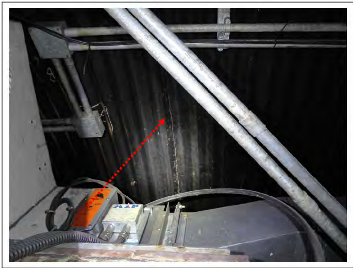
FIGURE 58: CONFIRMED ASBESTOS IN CELLACTITE SHEETING IN DISUSED, 6/401 - DESCRIPTION & RESULT OF ASSESSMENT (SAMPLE REF. AS ECS 85369)
