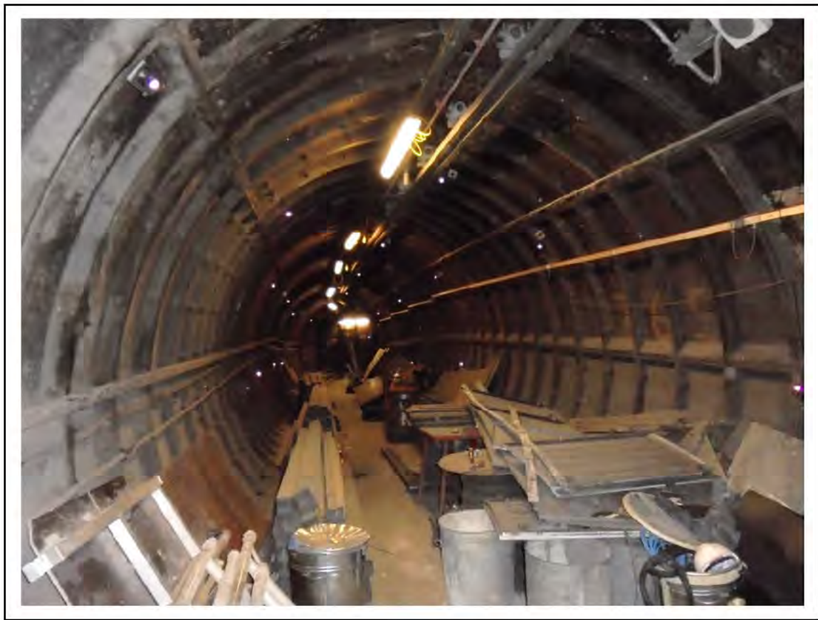
FIGURE 53: CONFIRMED ASBESTOS IN CAULKING TO TUNNEL RINGS IN DRAFT RELIEF TUNNEL, 6/792 - DESCRIPTION & RESULT OF ASSESSMENT (SAMPLE REF. 100675/110111/03)
