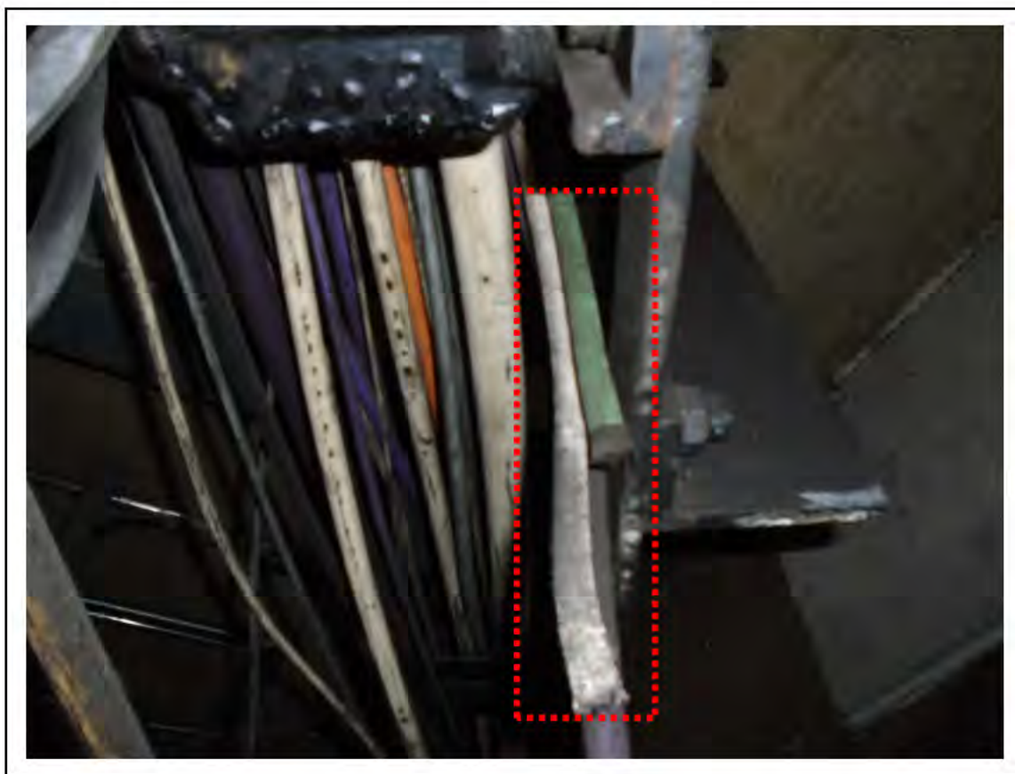
FIGURE 26: KNOWN ASBESTOS IN WOVEN CABLE INSULATION IN LMC 3, 4, 5, 6/161 - DESCRIPTION & RESULT OF ASSESSMENT (SAMPLE REF. K1 (2))
