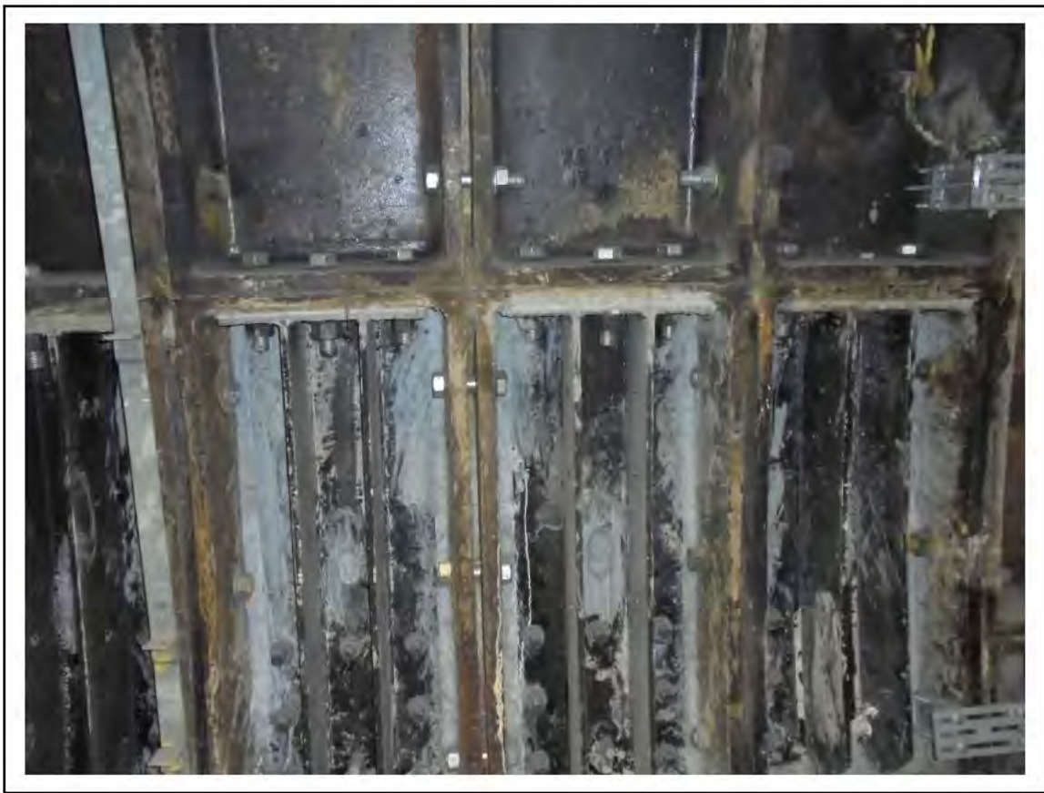
FIGURE 66: CONFIRMED ASBESTOS IN TUNNEL RING CAULKING IN CIRC AREA, 4/092 - DESCRIPTION & RESULT OF ASSESSMENT (SAMPLE REF. AS 014003/12)
