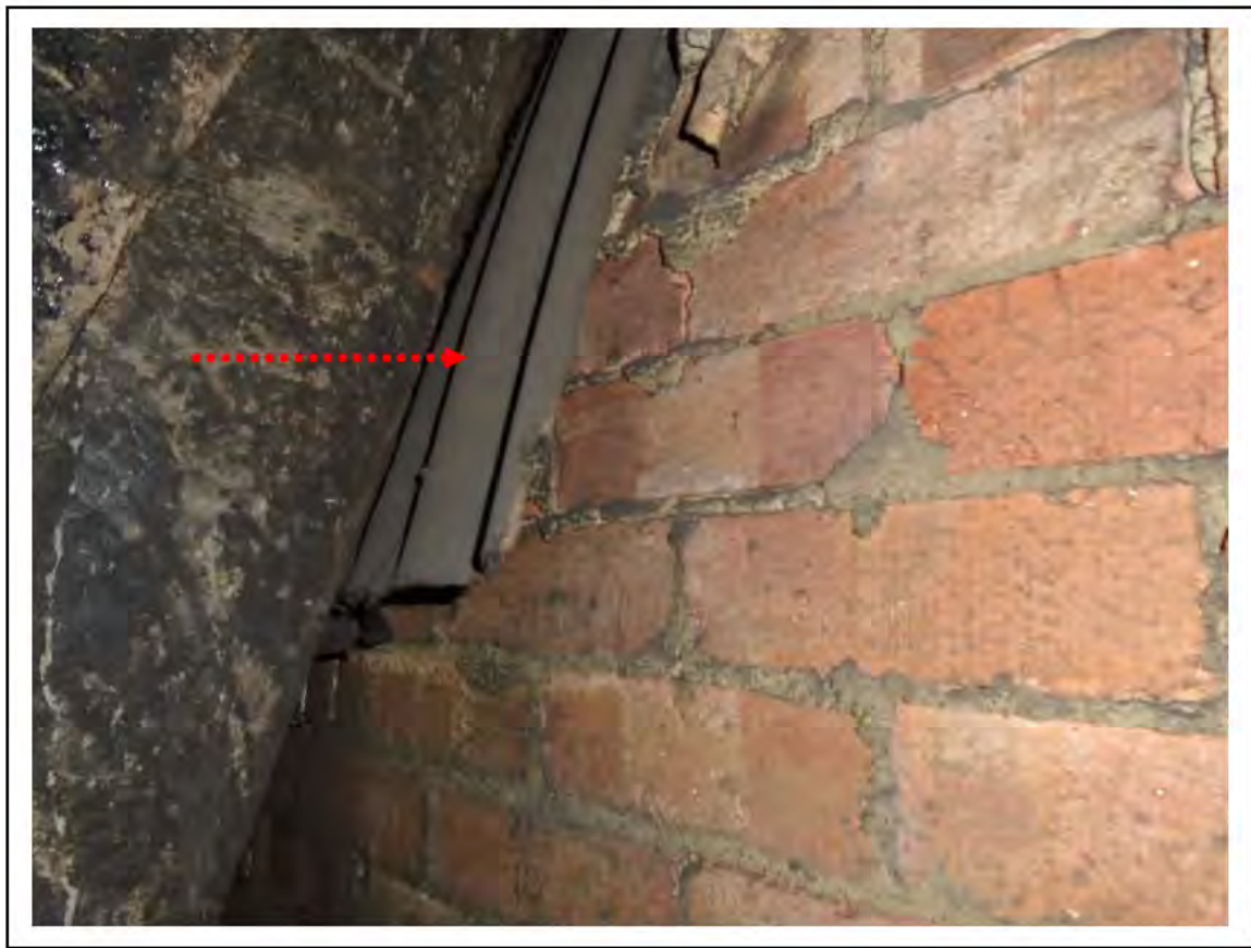
FIGURE 11: CONFIRMED ASBESTOS IN CELLACTITE SHEETING IN UMC 3, 4, 5 LOBBY TO CHAMBER, 4/161 - DESCRIPTION & RESULT OF ASSESSMENT (SAMPLE REF. 161057/220816/01)
