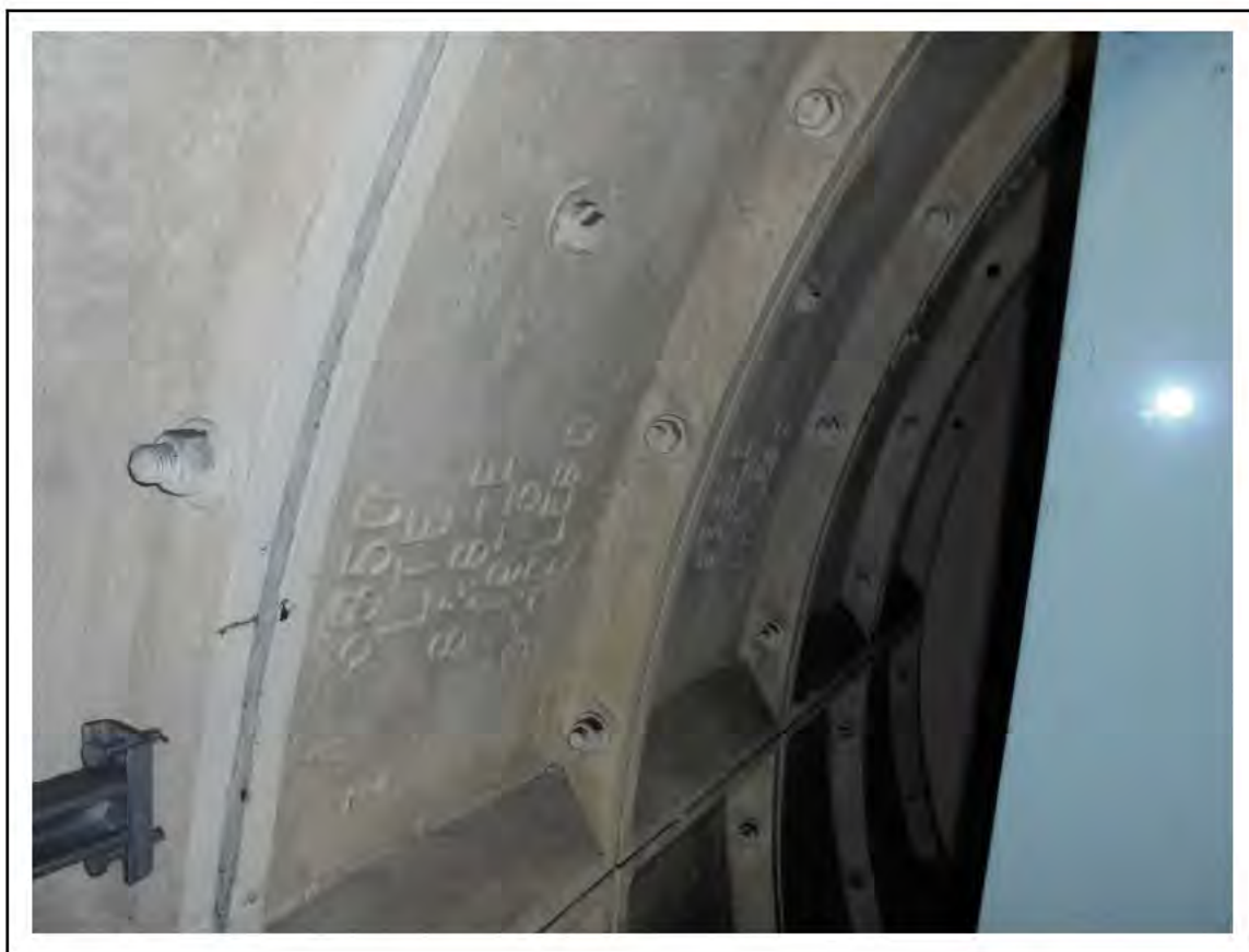
FIGURE 89: CONFIRMED ASBESTOS IN CAULKING IN SWITCH CUPBOARD E10, 6/663 - DESCRIPTION & RESULT OF ASSESSMENT (SAMPLE REF. ECS 85356)
