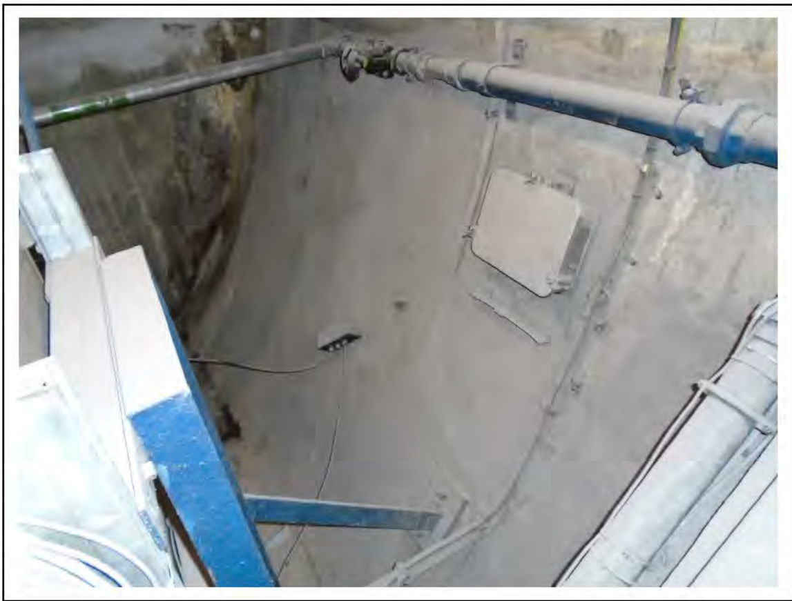
FIGURE 19: CONFIRMED ASBESTOS IN TUNNEL RING CAULKING IN LMC 6, 7, 8, 4/162 - DESCRIPTION & RESULT OF ASSESSMENT (SAMPLE REF. 110714/071111/01 & 02)
