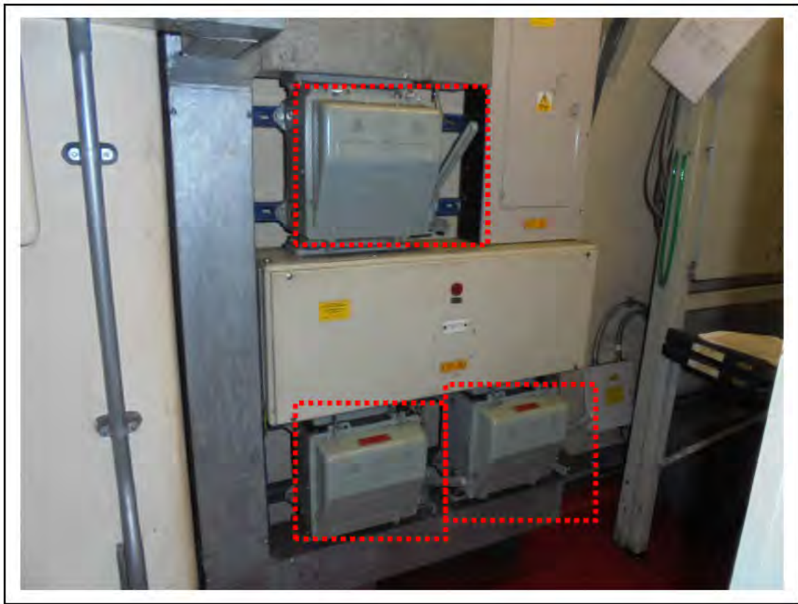
FIGURE 45: STRONGLY PRESUMED ASBESTOS IN COMBINATION FUSE SWITCHES IN SER, 4/711 - DESCRIPTION & RESULT OF ASSESSMENT (SAMPLE REF. SP1 (6))
