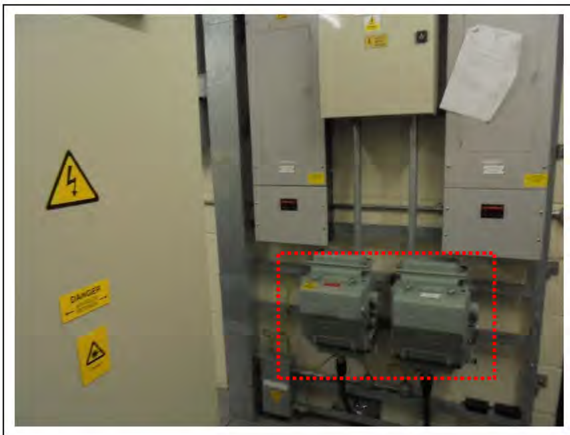
FIGURE 46: STRONGLY PRESUMED ASBESTOS IN COMBINATION FUSE SWITCHES IN CER, 4/731 - DESCRIPTION & RESULT OF ASSESSMENT (SAMPLE REF. SP1 (7))
