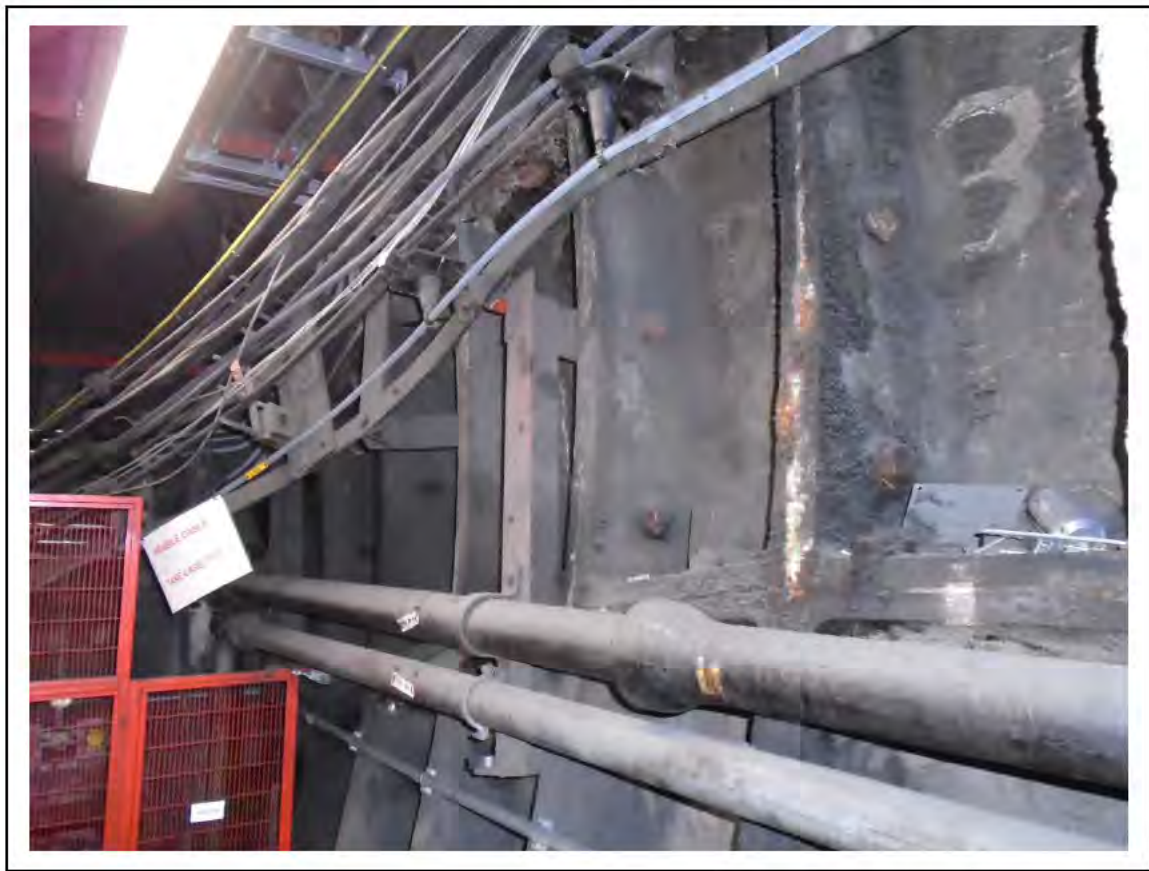
FIGURE 14: CONFIRMED ASBESTOS IN TUNNEL RING CAULKING IN UMC 3,4,5, 4/161 - DESCRIPTION & RESULT OF ASSESSMENT (SAMPLE REF. 100558/121010/16)
