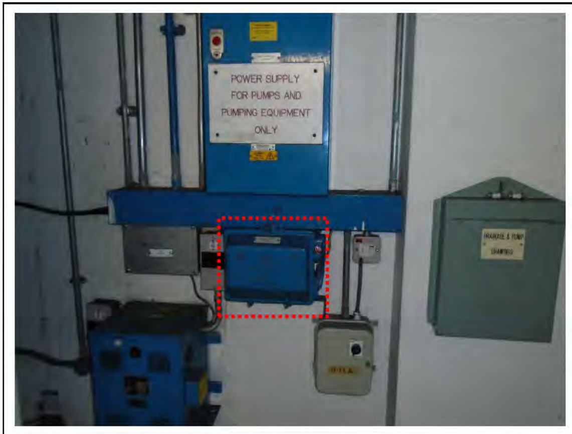
FIGURE 9: STRONGLY PRESUMED ASBESTOS IN MATERIALS WITHIN COMBINATION FUSE SWITCH IN PUMP ROOM, 3/771 - DESCRIPTION & RESULT OF ASSESSMENT (SAMPLE REF. SP1 (2))
