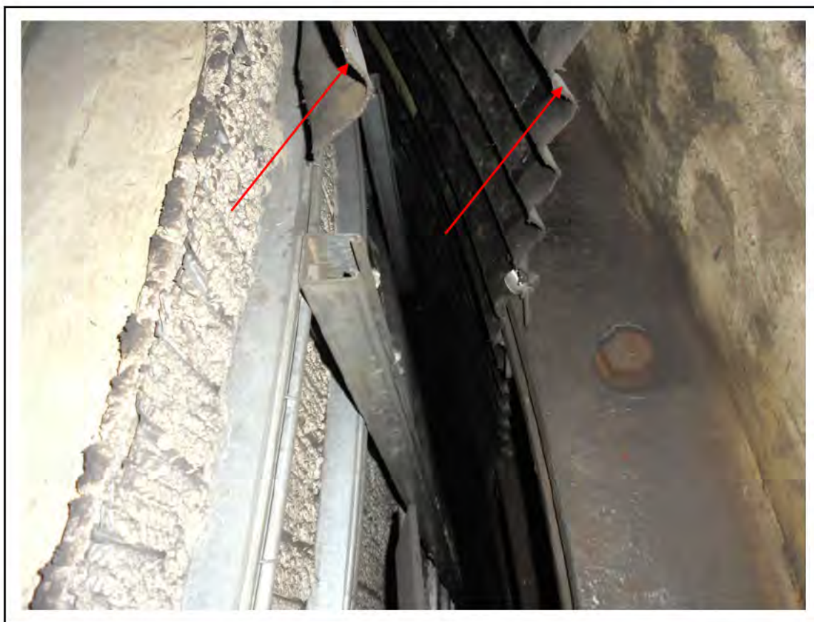
FIGURE 60: KNOWN ASBESTOS IN CELLACTITE SHEETING IN FLAMMABLE STORE, 6/901 - DESCRIPTION & RESULT OF ASSESSMENT (SAMPLE REF. K1 (8))
