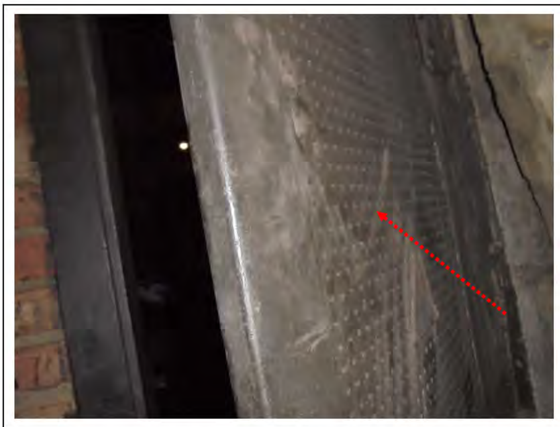
FIGURE 38: CONFIRMED ASBESTOS IN DURASTEEL PANEL IN CABLE TUNNEL, 4/787 - DESCRIPTION & RESULT OF ASSESSMENT (SAMPLE REF. ECS 76822)
