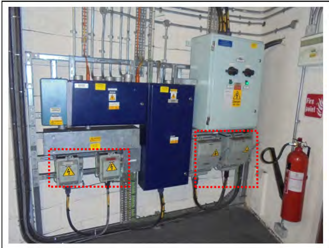
FIGURE 48: STRONGLY PRESUMED ASBESTOS IN MATERIALS WITHIN COMBINATION FUSE SWITCHES IN SWITCH ROOM, 4/763 - DESCRIPTION & RESULT OF ASSESSMENT (SAMPLE REF. SP1 (8))
