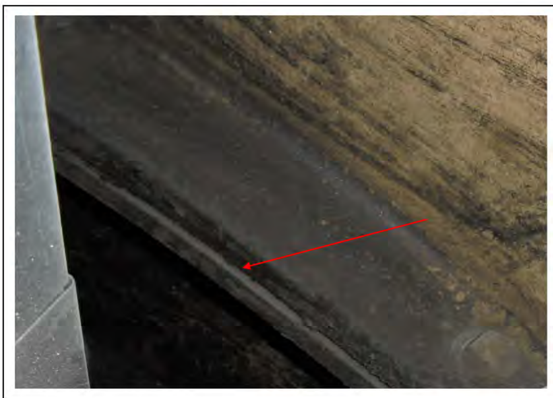
FIGURE 62: CONFIRMED ASBESTOS IN TUNNEL RING CAULKING IN OVERBRIDGE AND PASSAGE, 4/638 - DESCRIPTION & RESULT OF ASSESSMENT (SAMPLE REF. SAME AS ECS 85377)
