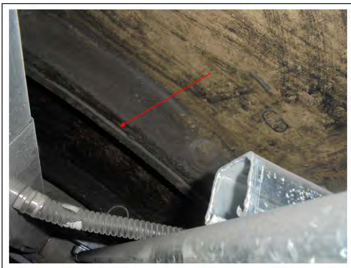
FIGURE 65: CONFIRMED ASBESTOS IN TUNNEL RING CAULKING IN PASSAGE AND OVERBRIDGE, 4/206 & 4/639 - DESCRIPTION & RESULT OF ASSESSMENT (SAMPLE REF. 100675/100211/01)
