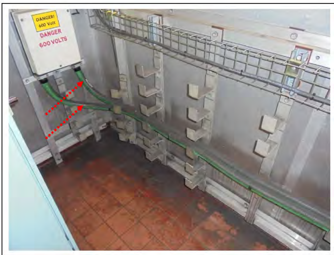
FIGURE 88: KNOWN ASBESTOS IN WOVEN CABLE INSULATION IN CER, 6/714 - DESCRIPTION & RESULT OF ASSESSMENT (SAMPLE REF. K1 (12))
