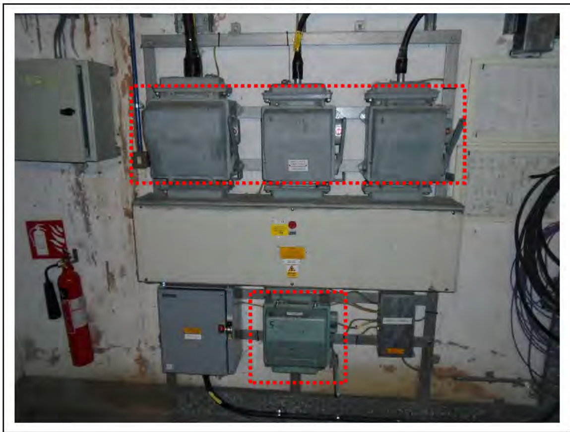
FIGURE 17: STRONGLY PRESUMED ASBESTOS IN COMBINATION FUSE SWITCHES IN SWITCHROOM E4, 2/664 - DESCRIPTION & RESULT OF ASSESSMENT (SAMPLE REF. SP1 (4))
