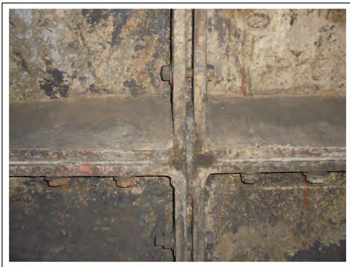
FIGURE 35: CONFIRMED ASBESTOS IN CAULKING IN CABLE TUNNEL, 4/786 - DESCRIPTION & RESULT OF ASSESSMENT (SAMPLE REF. ECS 85379)
