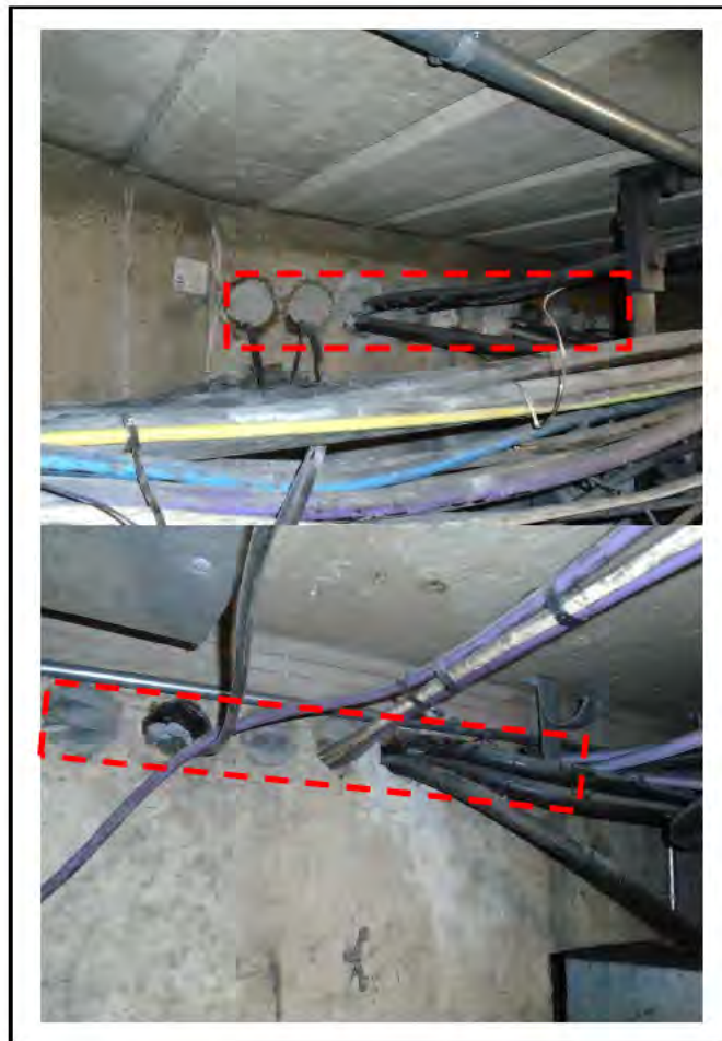
FIGURE 30: CONFIRMED ASBESTOS IN BITUMEN DUCTS IN LMC 3, 4, 5 CRAWLWAY, 6/161 - DESCRIPTION & RESULT OF ASSESSMENT (SAMPLE REF. 161144/190916/01-10 & 12-18)
