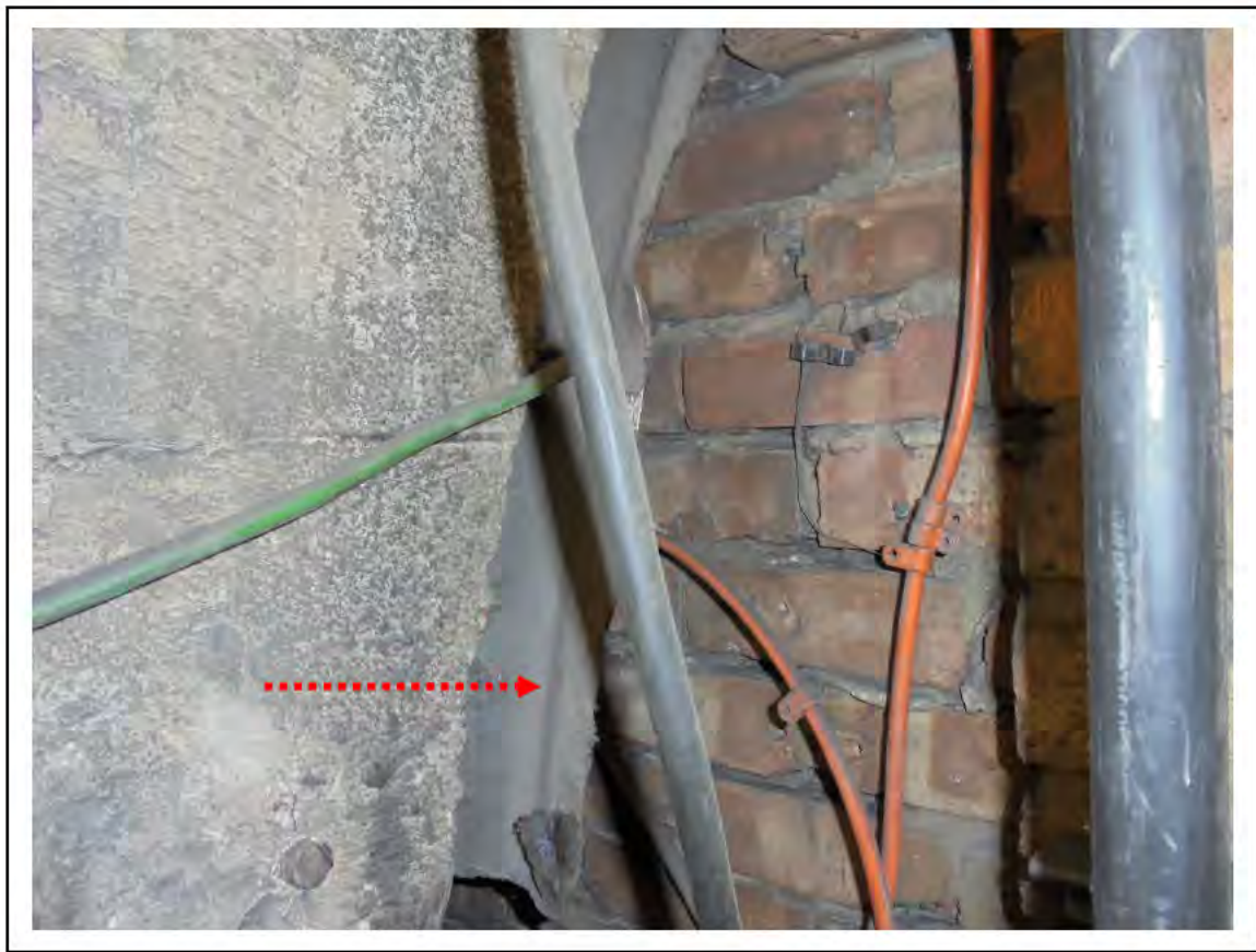
FIGURE 83: CONFIRMED ASBESTOS IN CELLACTITE SHEETING IN BOSTWICK GATE CHAMBER, 4/765 - DESCRIPTION & RESULT OF ASSESSMENT (SAMPLE REF. 161057/011216/01)
