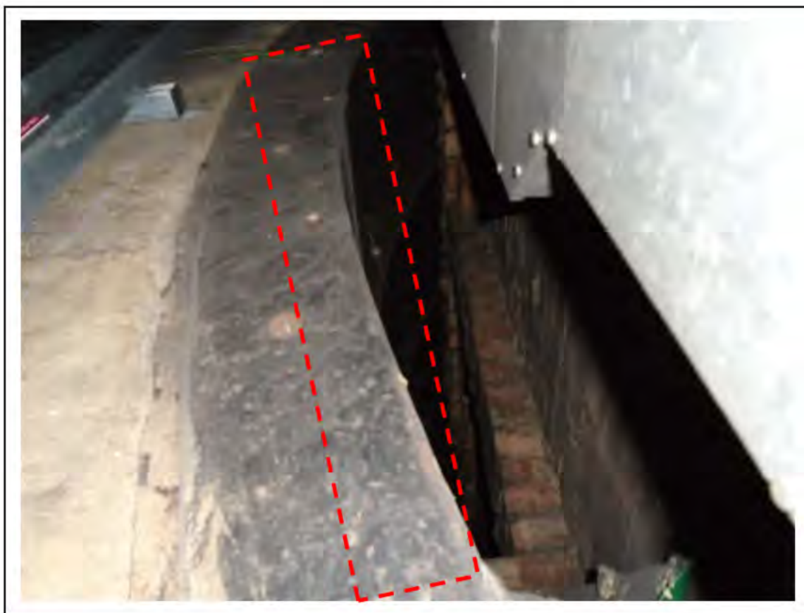
FIGURE 23: CONFIRMED ASBESTOS IN TUNNEL RING CAULKING IN LMC 3, 4, 5 LOBBY, 6/161 - DESCRIPTION & RESULT OF ASSESSMENT (SAMPLE REF. AS 100558/141010/1)
