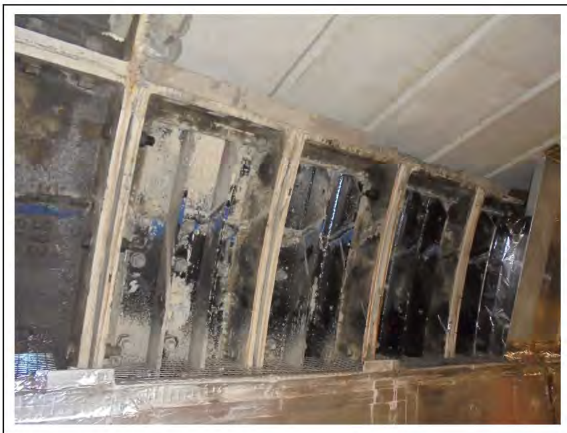
FIGURE 76: CONFIRMED ASBESTOS IN TUNNEL RING CAULKING IN PLATFORM 4, 6/262 - DESCRIPTION & RESULT OF ASSESSMENT (SAMPLE REF. 110103/150511/01 & 02)
