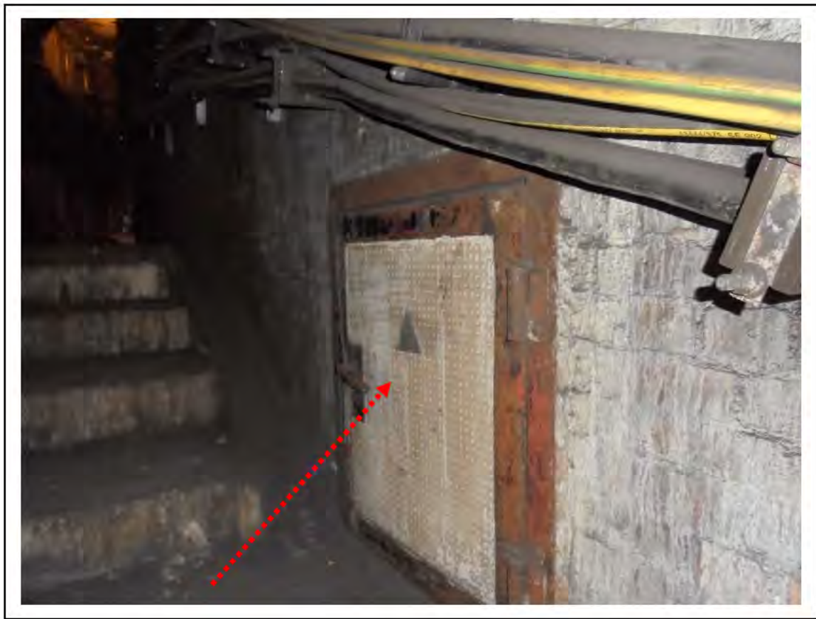
FIGURE 41: CONFIRMED ASBESTOS IN DURASTEEL PANEL IN CABLE TUNNEL, 4/787 - DESCRIPTION & RESULT OF ASSESSMENT (SAMPLE REF. 014003/18)
