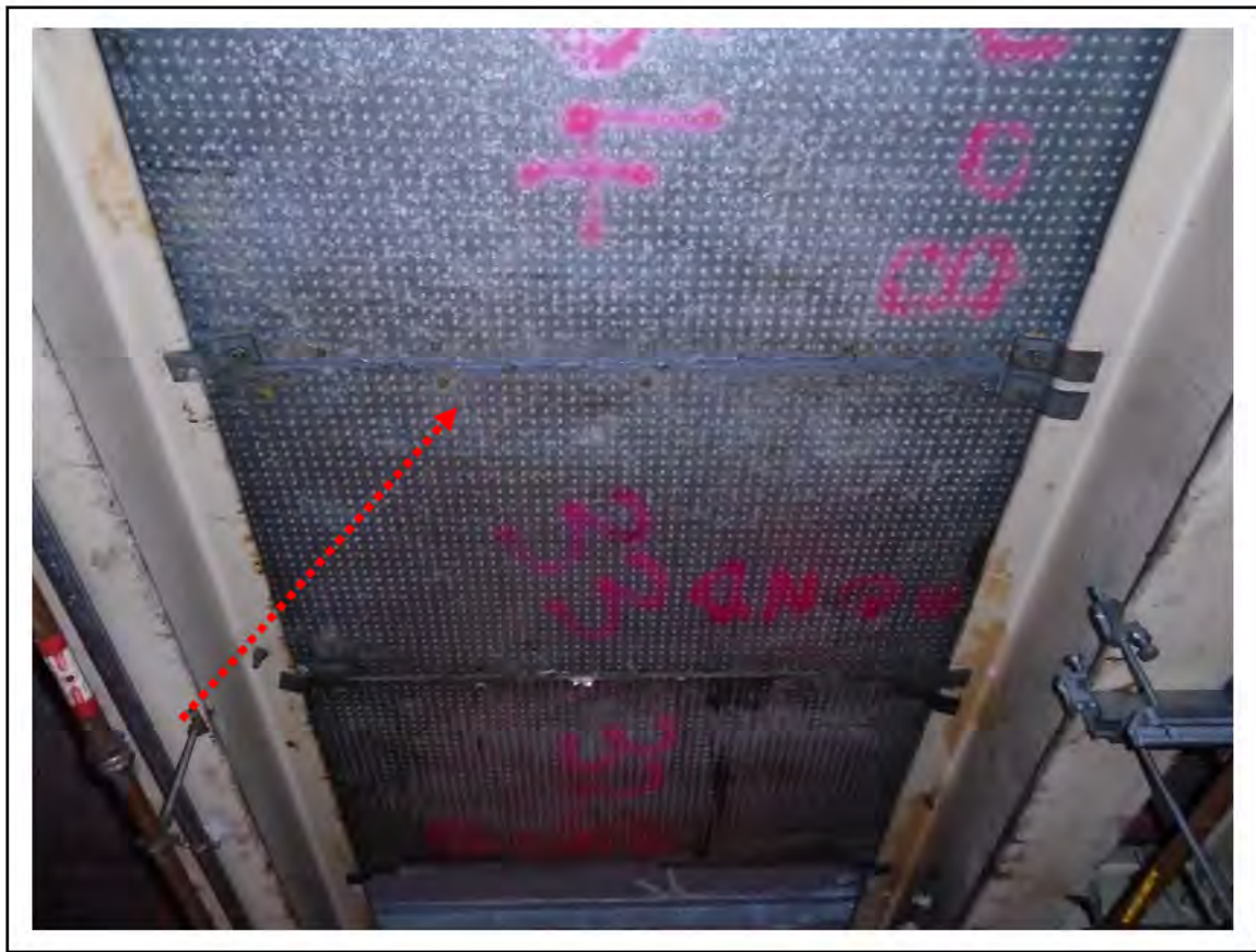
FIGURE 15: CONFIRMED ASBESTOS IN DURASTEEL PANELS IN UMC 3, 4, 5, 4/161 - DESCRIPTION & RESULT OF ASSESSMENT (SAMPLE REF. 161057/220816/02)
