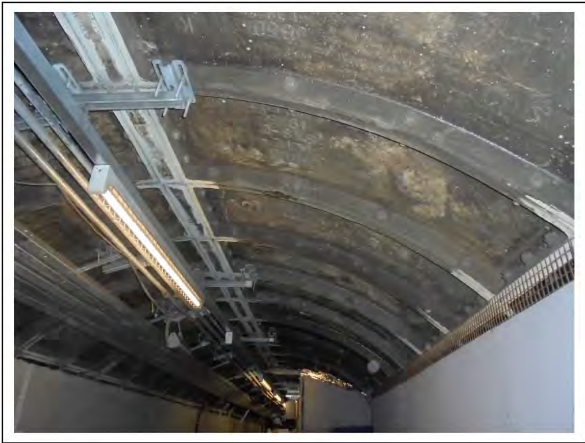
FIGURE 56: KNOWN ASBESTOS IN CAULKING TO TUNNEL RINGS IN PASSAGE, 6/201 - DESCRIPTION & RESULT OF ASSESSMENT (SAMPLE REF. K1 (7))
