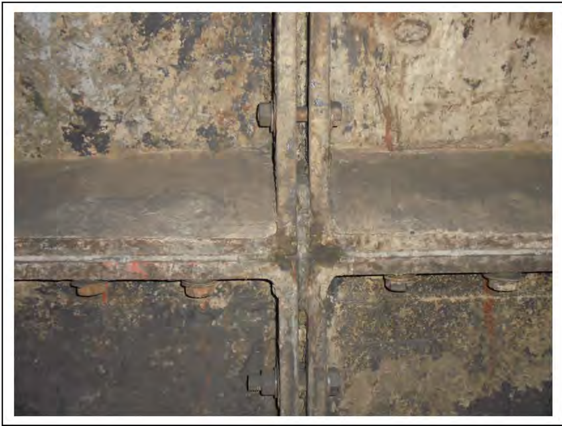
FIGURE 42: KNOWN ASBESTOS IN CAULKING IN CABLE RUN SHAFT, BY END OF CABLE TUNNEL 4/787 - DESCRIPTION & RESULT OF ASSESSMENT (SAMPLE REF. K1 (5))
