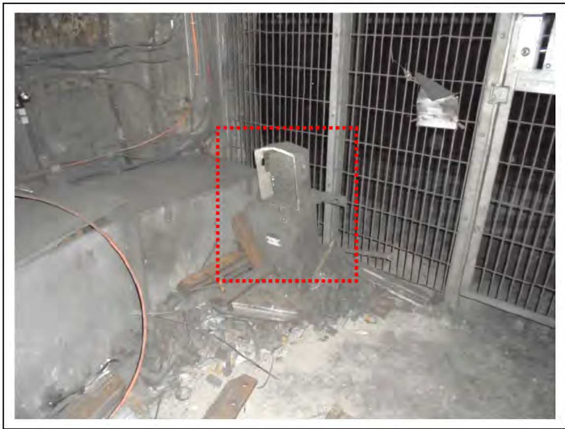
FIGURE 54: PRESUMED ASBESTOS IN MATERIALS WITHIN WESTINGHOUSE BOXES IN DRAFT RELIEF TUNNEL, 6/792 - DESCRIPTION & RESULT OF ASSESSMENT (SAMPLE REF. P1 (1))
