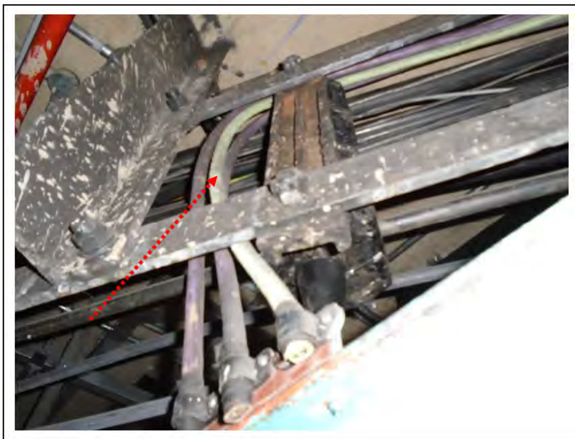
FIGURE 25: KNOWN ASBESTOS IN WOVEN CABLE INSULATION IN LMC 3, 4, 5, 6/161 - DESCRIPTION & RESULT OF ASSESSMENT (SAMPLE REF. K1 (1))
