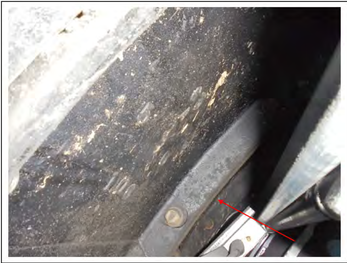
FIGURE 61: CONFIRMED ASBESTOS IN TUNNEL RING CAULKING IN INTERMEDIATE CONCOURSE, 4/203 - DESCRIPTION & RESULT OF ASSESSMENT (SAMPLE REF. ECS 85377)
